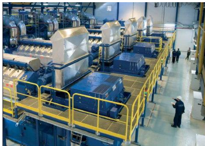
10 MWe gas CHP engines
